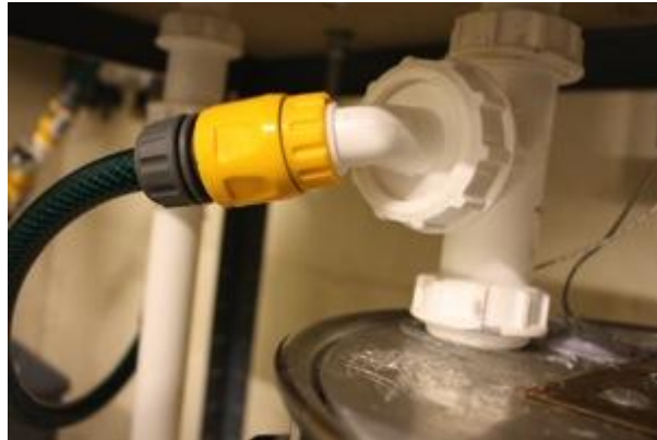
Figure 10.3: Water Inlet Connection to the Vessels.
